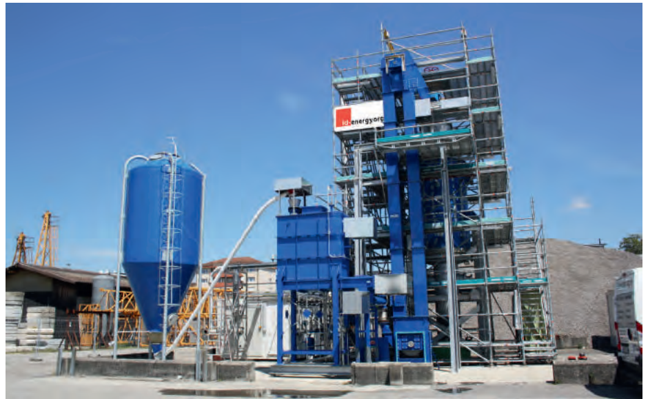
TCC Educator Anlage in Zofingen
