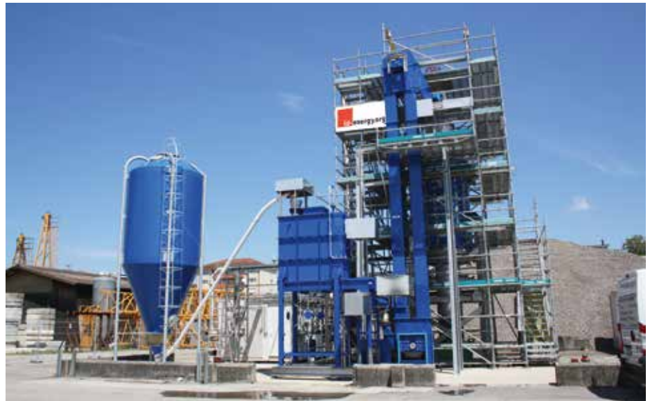
TCC Educator Anlage in Zofingen
