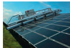
GEKKO Solar Farm
