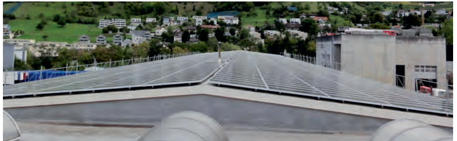
Photovoltaik Anlage 170 kWp
