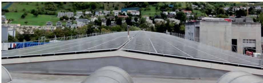
Photovoltaik Anlage 170 kWp
