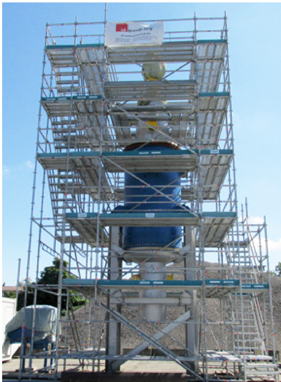
Educator Anlage in Zofingen
