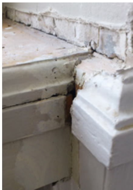
Fenstersimse vor Renovation.
